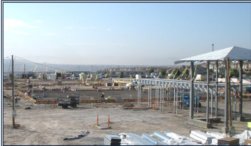
Building 300 preparation prior to pouring slab. Tower of Building 100 and walkway are on the right. ↓
